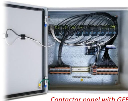
Contactor panel with GFEP
