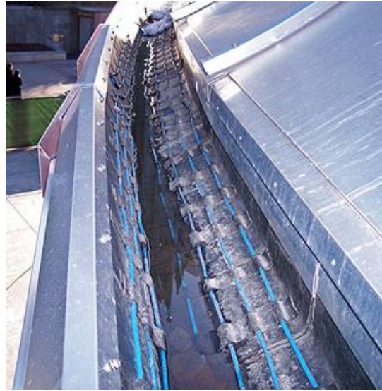
Heat cable installed for commercial gutter heat trace system (SLC Tabernacle)
