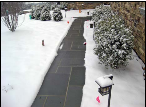
ClearZone snow melting system installed under paver sidewalk.
