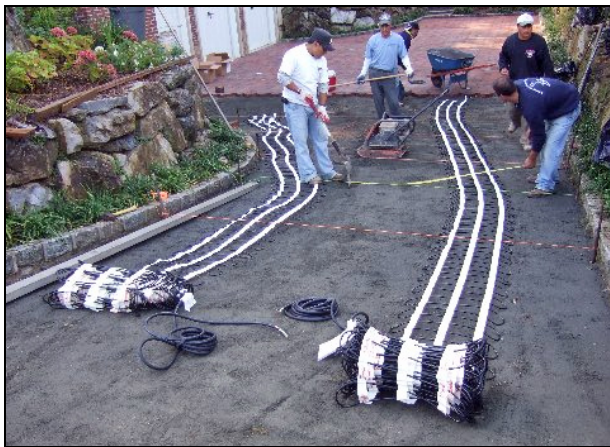
ClearZone snow melting mats being installed for heated paver tire track driveway.
