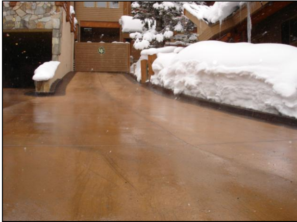
ClearZone system installed in stained concrete.
