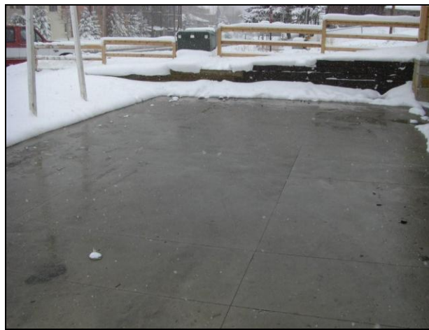
CZ-heated concrete driveway and parking area.
